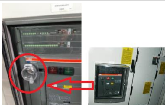
Envolvente instalada sobre el bombín del interruptor/ Plastic cover installed on the cylinder in the Circuit breaker.
